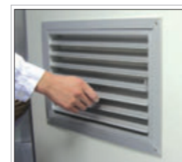
Adjustable air flow vents in each work area.
