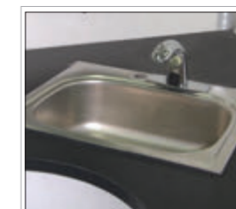
Stainless steel sink with hands-free water faucet.
