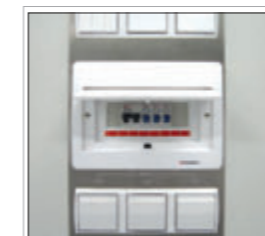
Switch and circuit breaker panel are centrally located
